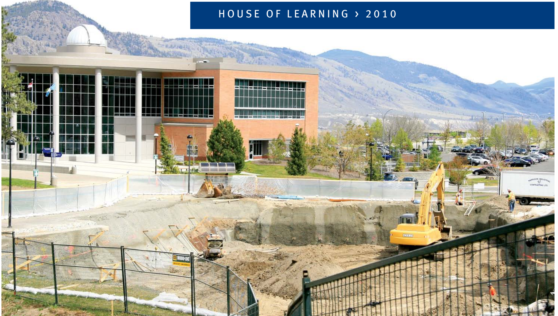
Construction crews hollow out the earth for the House of Learning. The International Building stands behind it to the left. Photo – Bart Cummins
