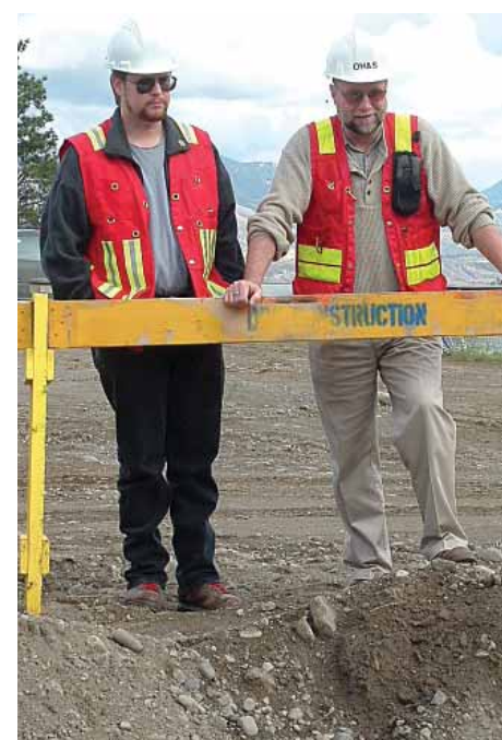
David Graham, a contractor, and Doug Sweeney of TRU inspect an open trench at the natural resource science greenhouse construction site.
